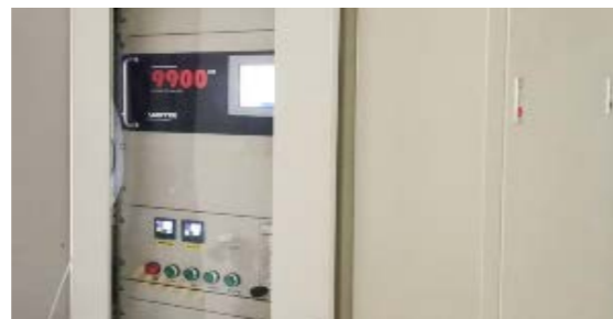
Upgrading the Flue Gas Online Monitoring System at Asia Symbol (Jiangsu)
